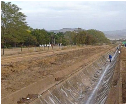
Photo 6: Irrigation canal Pongola: Before
